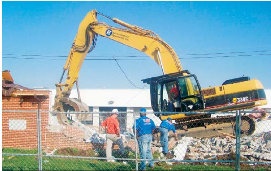
Construction workers tearing down an old building to make room for new dormitories.
