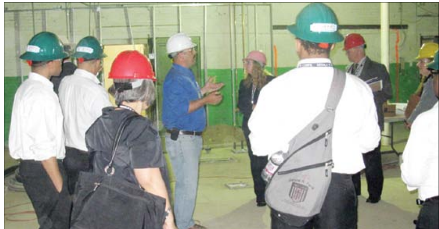
In the photo above, John Brondsema (center) Superintendent of Nevilles Electric Service explains renovations to representatives from the Department of Labor, the Student Government Association and Gerald R. Ford Job Corps Center staff members.
